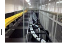
Cable Ladder inside the Server Room
